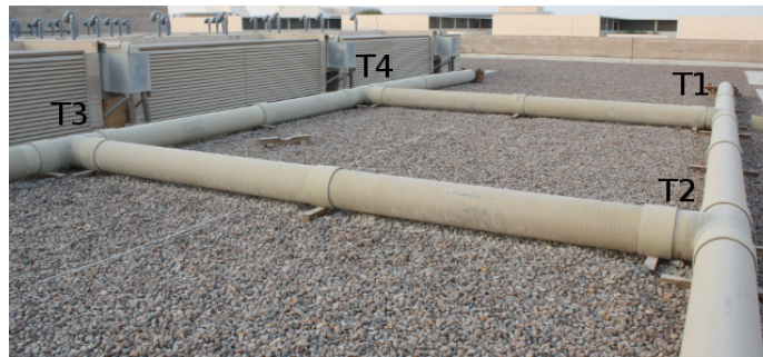
(c) The pipe network with labeled T-intersections for reference. Observe that each of the long straight sections is constructed from two straight segments of pipe.
